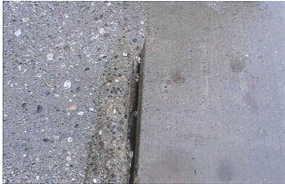
CK2378 Right ballast wall damage
